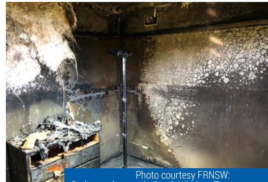
Photo courtesy FRNSW: Bedroom damage in South Windsor Fire.
